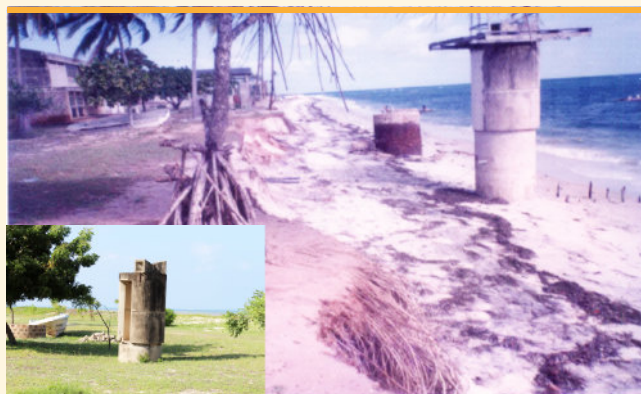
Seawater pumping station and a watchtower of the Kunduchi Marine Biology Station as they appeared being threatened by the beach erosion in December 1995 and current situation (the insert). ©Albogast T. Kamukuru
